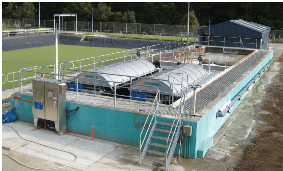
Two Forty-X disc filters were retrofitted to a wastewater facility in New Zealand to increase plant capacity. Image courtesy of Siemens Water Technologies.
